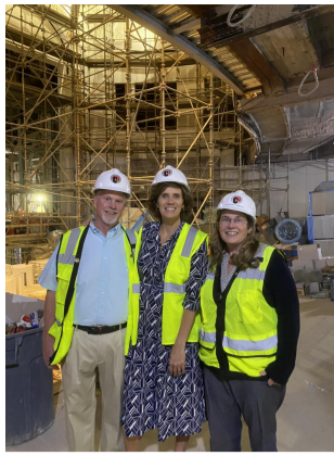
I had a great tour of the massive renovation happening at the Carolina Theatre in uptown Charlotte recently. I'm looking forward to seeing the completed facility once construction is complete.
